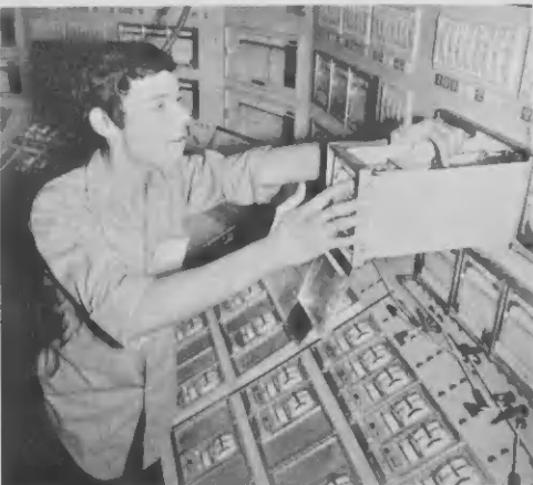
Assigned to Instrument Section, electrical student Mariano Arends observes intricate panel recorder box at the Refining Control Center.
